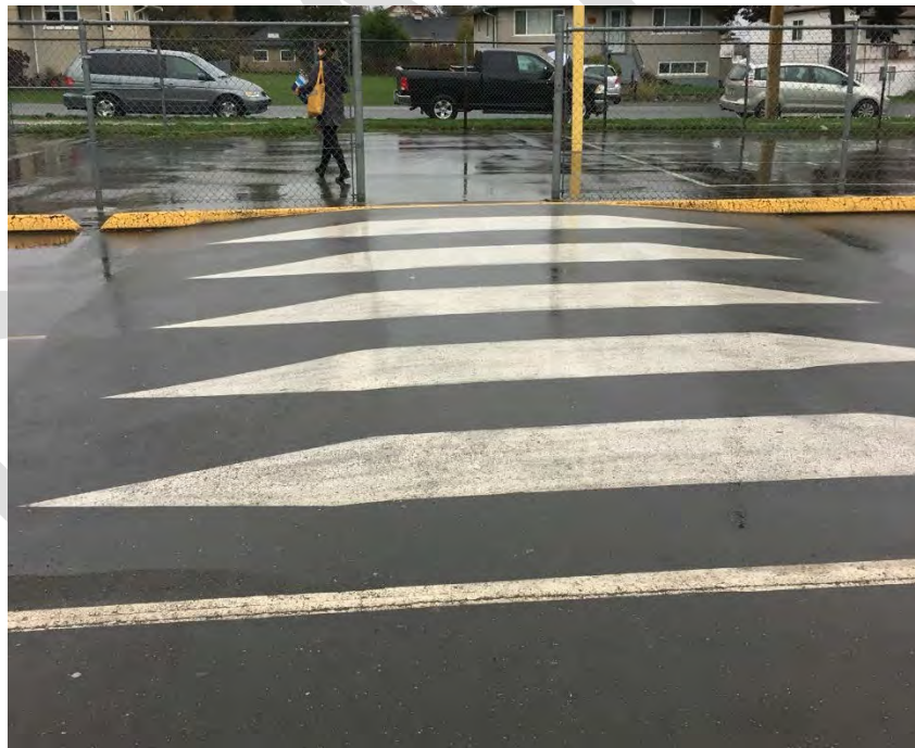
Figure 12 - Speed bump - part of pedestrian path from basketball court
